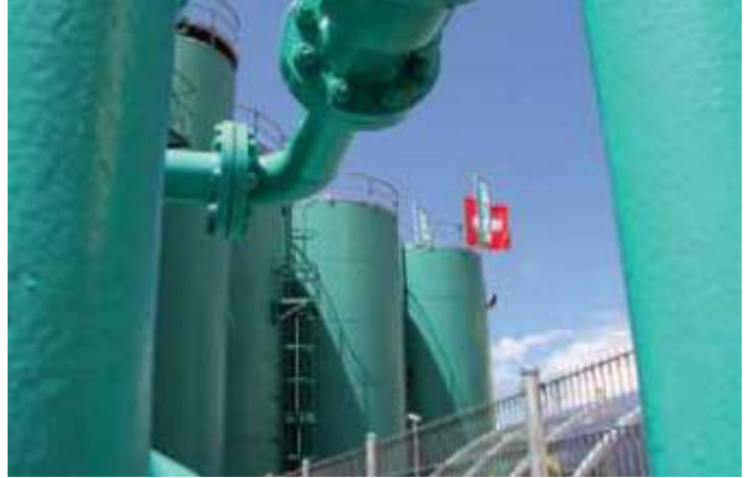
The tank facilities are an important component of the precisely defined extensive production procedures carried out by Motorex in accordance with ISO standards.
